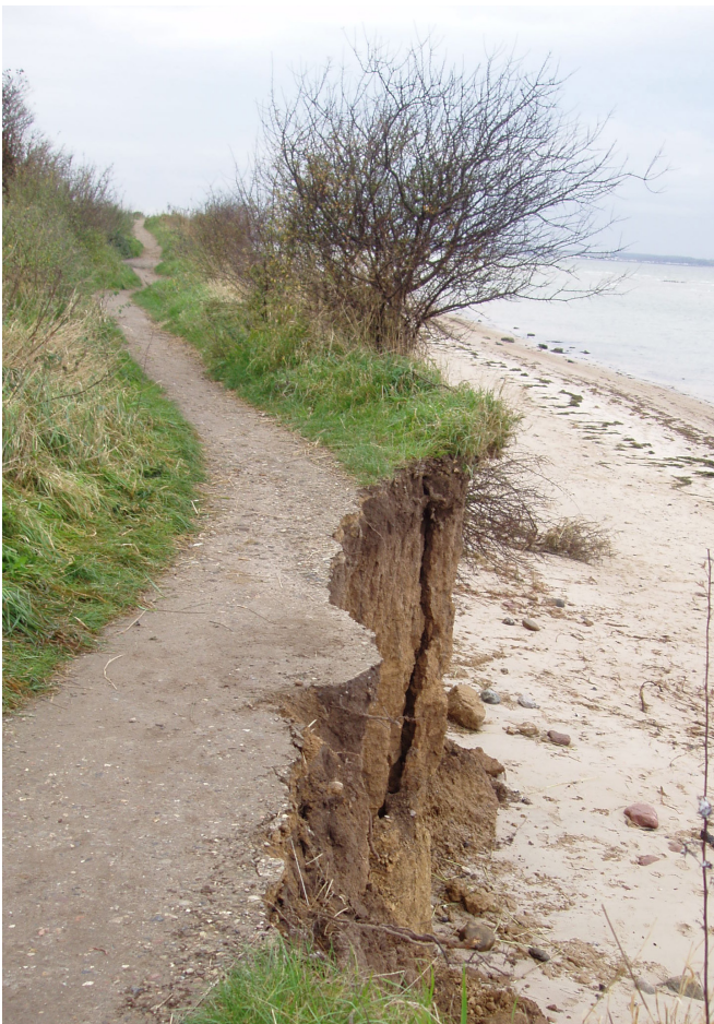
Accelerated erosion near Baltic coastline results in damage to infrastructure. Credit: Horst Sterr
